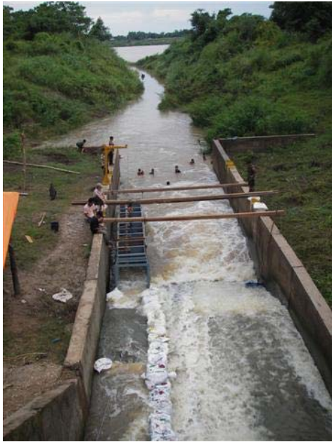
Upstream view of the fishway. The sandbag wall was used to control flows through the structure
